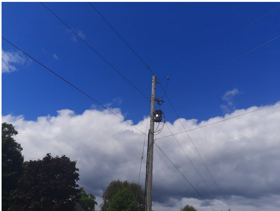
Photo 12 Pole-mounted oil-cooled transformer east of the Site (PCA), September 7, 2022.
