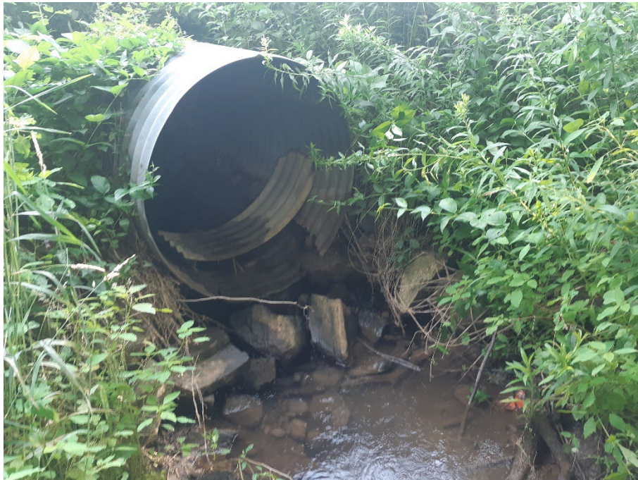
Photo 2 Perched culvert outlet on Ganaraska Road, July 2021.
